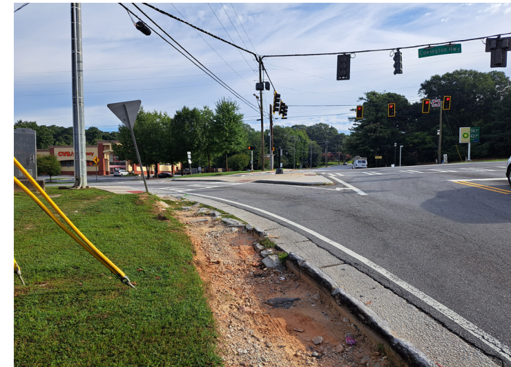
MISSING CONNECTION BETWEEN RAMP AND SIDEWALK AT COVINGTON HIGHWAY
