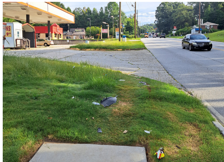
SIDEWALK ABRUPTLY ENDS ON WEST SIDE, BUS STOP WITH NO SIDEWALK OR CONCRETE PAD
