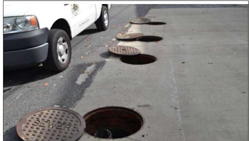
DeKalb County Water Mains
