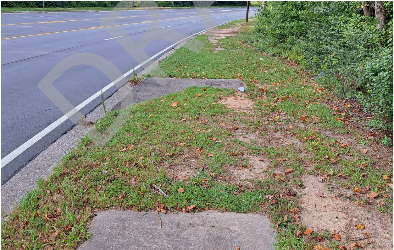
Sidewalk Gap on Mall Parkway Near Honeycreek Court
