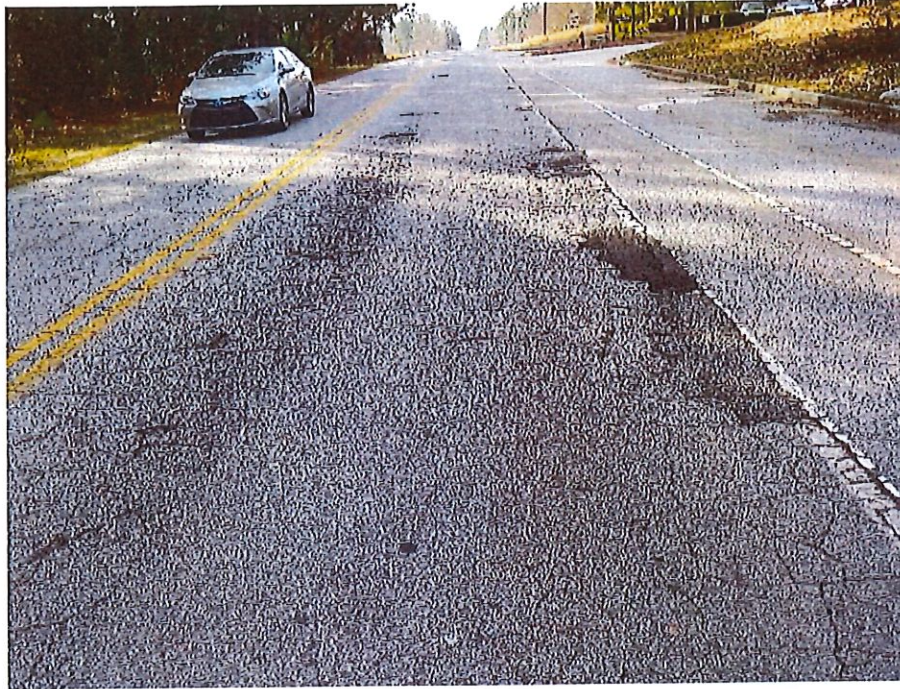
Level 4 load cracking, Southbound, Lane 1, Station 15+00±
