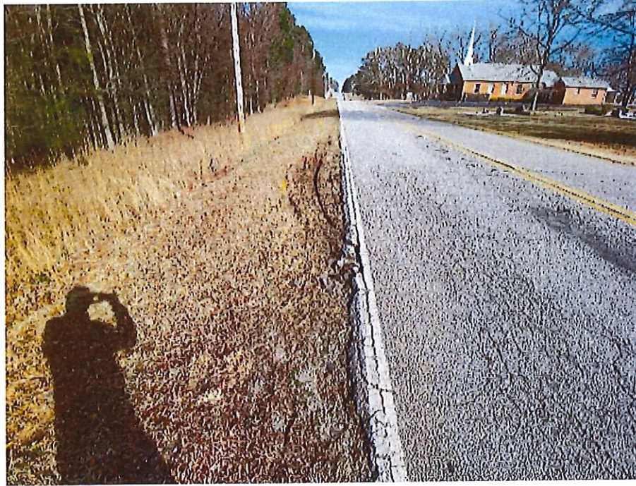
Level 3 Edge Distress, Southbound, Station 29+50±
