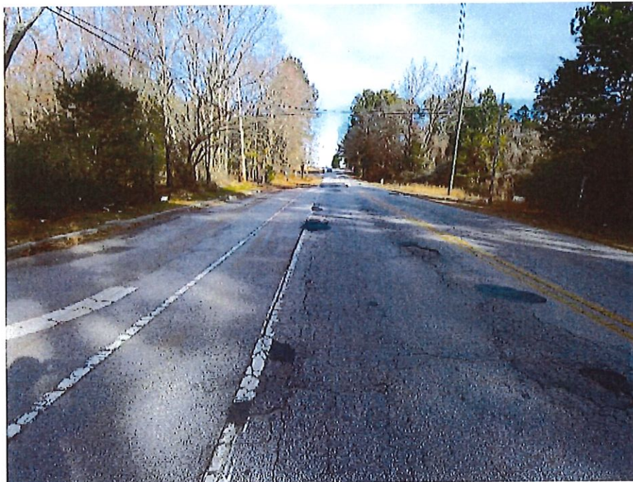
Patch/ Potholes, Southbound, Lane 1, Station 14+00±
