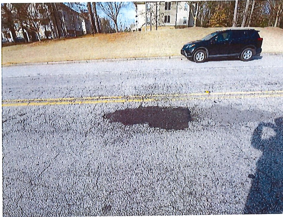
Patch/ Pothole, Northbound, Lane 1, Station 16+00±
