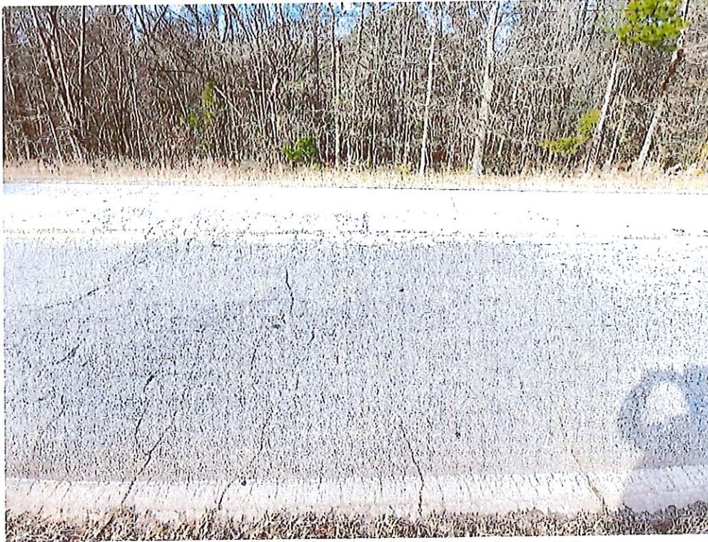
Level 2 block cracking, Northbound, Lane 1, Station 24+50±
