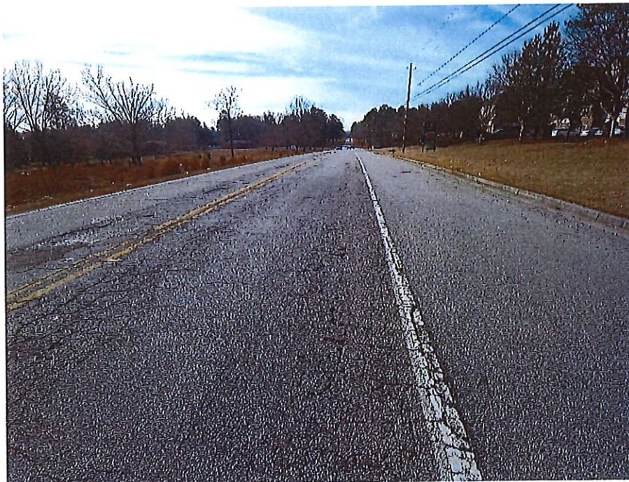
Level 4 load cracking, Southbound, Lane 1, Station 16+00±
