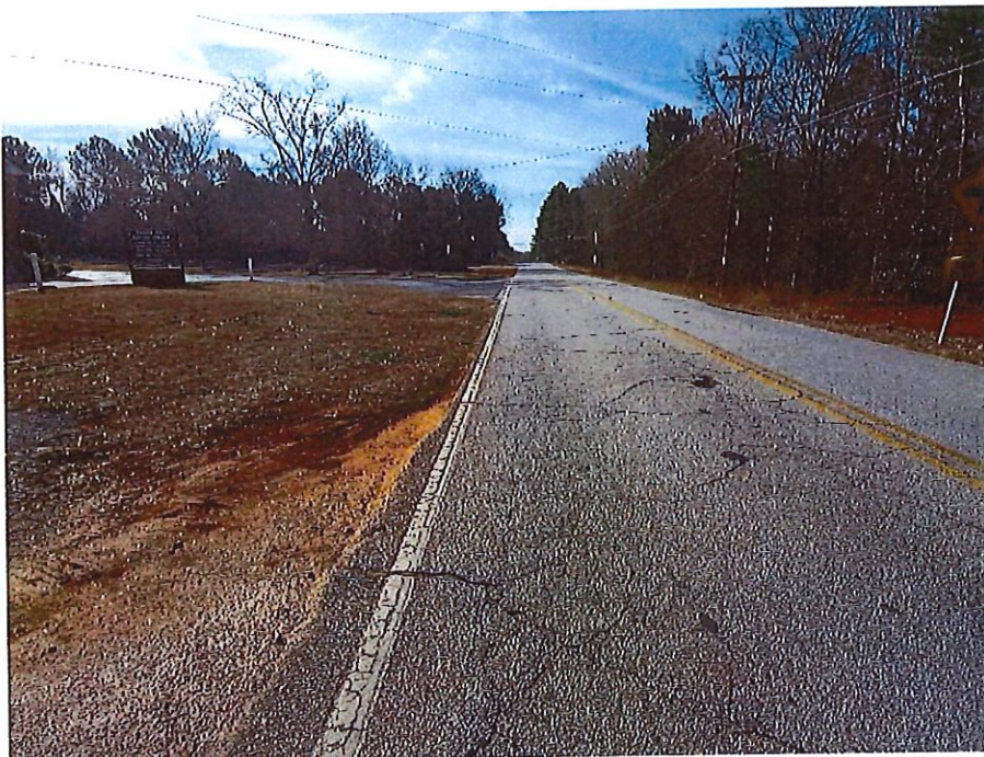
Level 3 load cracking, Northbound, Lane 1, Station 25+50±
