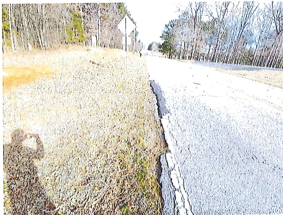
Level 3 Edge Distress, Southbound, Station 27+50±
