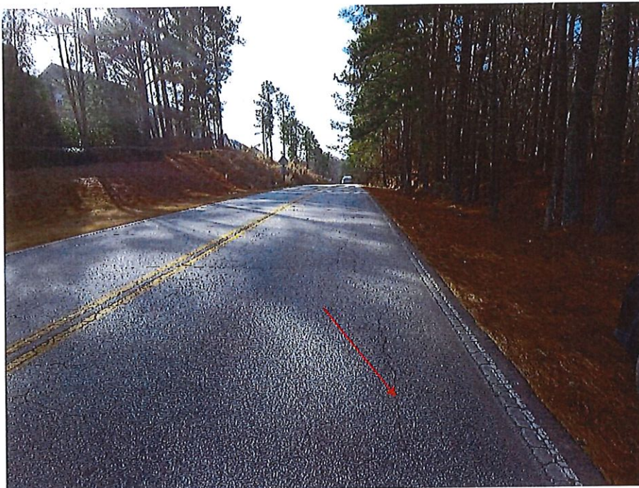
Level 1 load cracking, Northbound, Lane 1, Station 44+00±
