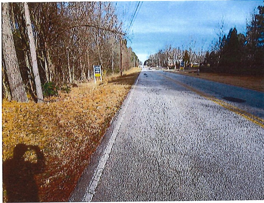
Level 3 load cracking, Southbound, Lane 1, Station 36+50±
