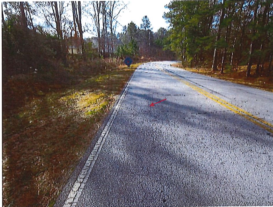
Level 2 load cracking, Northbound, Lane 1, Station 42+00±
