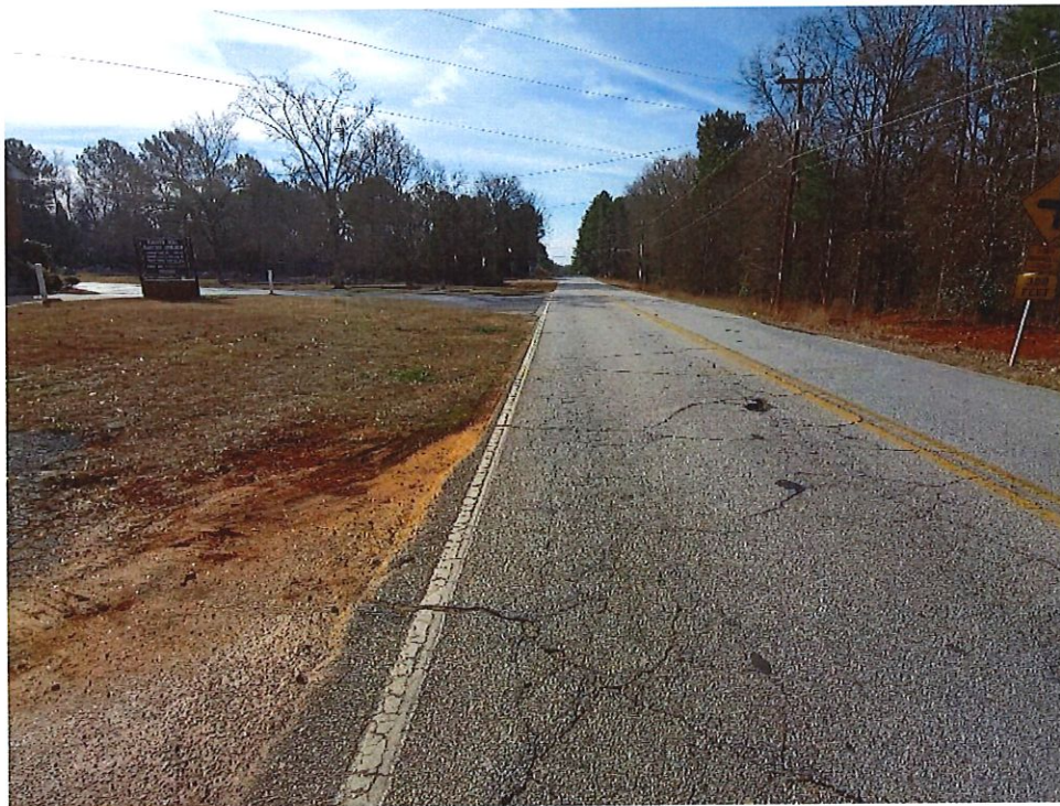
Level 3 load cracking, Northbound, Lane 1, Station 25+50±
