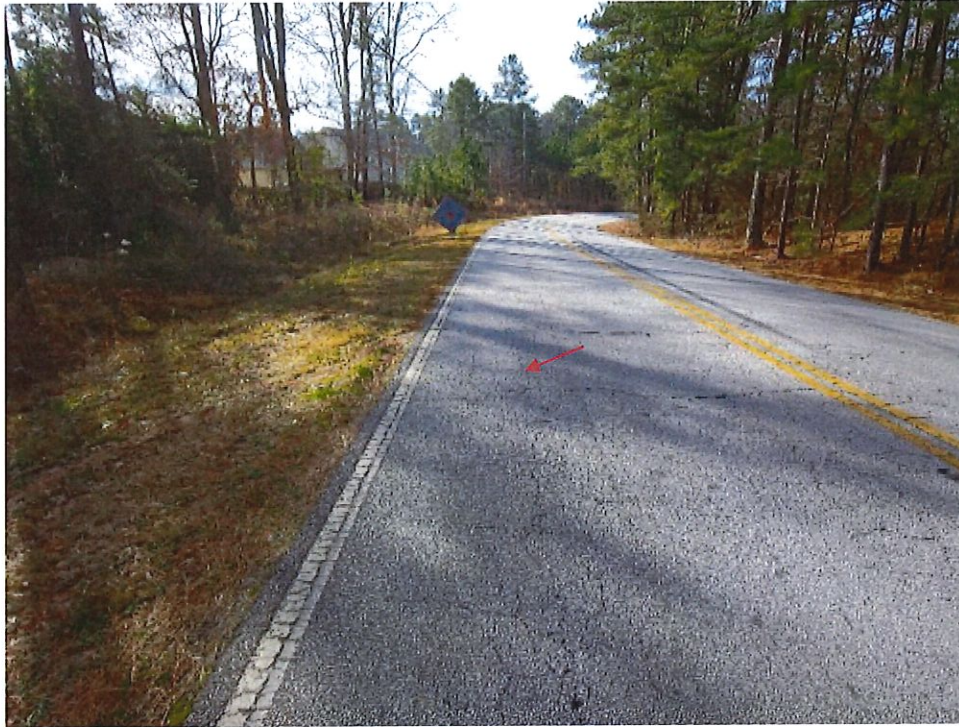
Level 2 load cracking, Northbound, Lane 1, Station 42+00±
