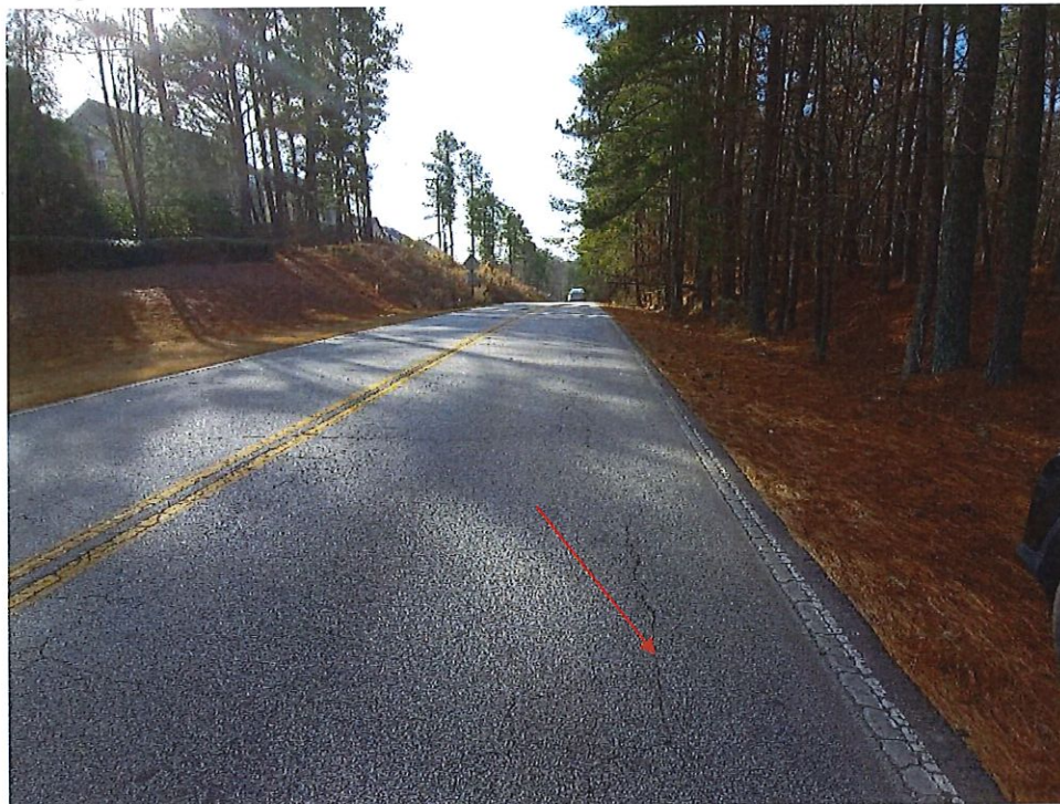
Level 1 load cracking, Northbound, Lane 1, Station 44+00±
