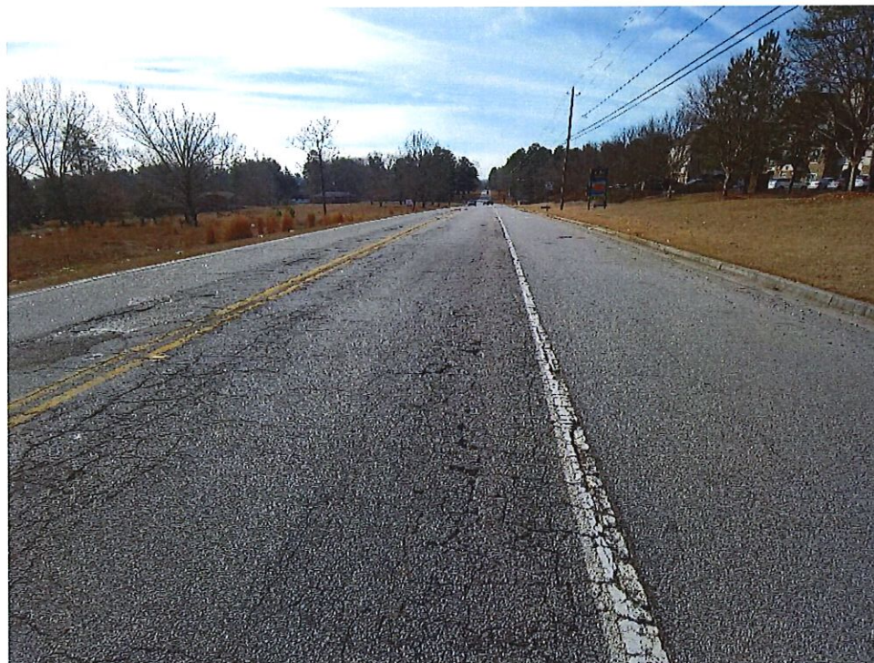
Level 4 load cracking, Southbound, Lane 1, Station 16+00±
