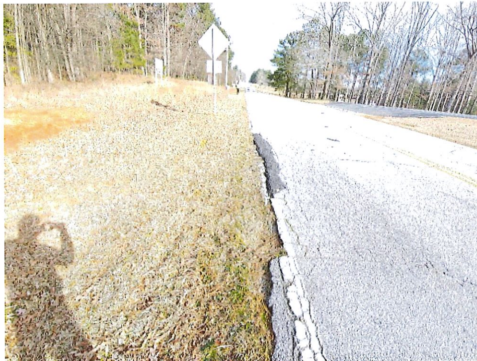
Level 3 Edge Distress, Southbound, Station 27+50±
