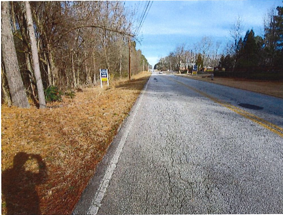
Level 3 load cracking, Southbound, Lane 1, Station 36+50±
