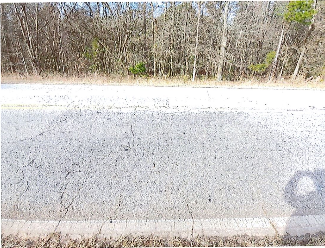
Level 2 block cracking, Northbound, Lane 1, Station 24+50±
