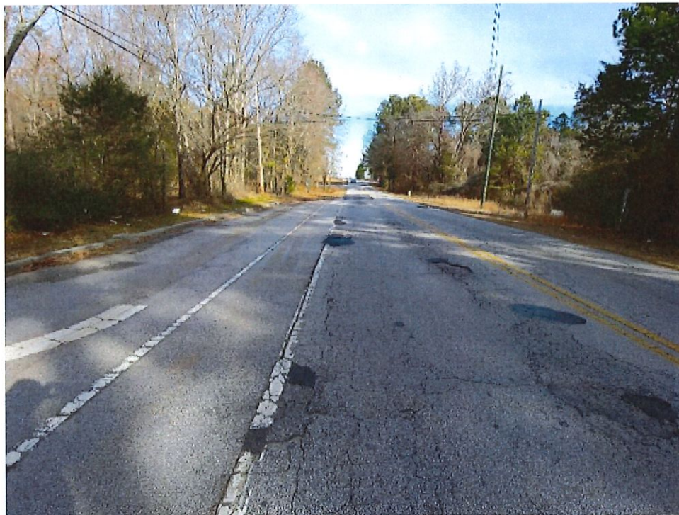
Patch/ Potholes, Southbound, Lane 1, Station 14+00±
