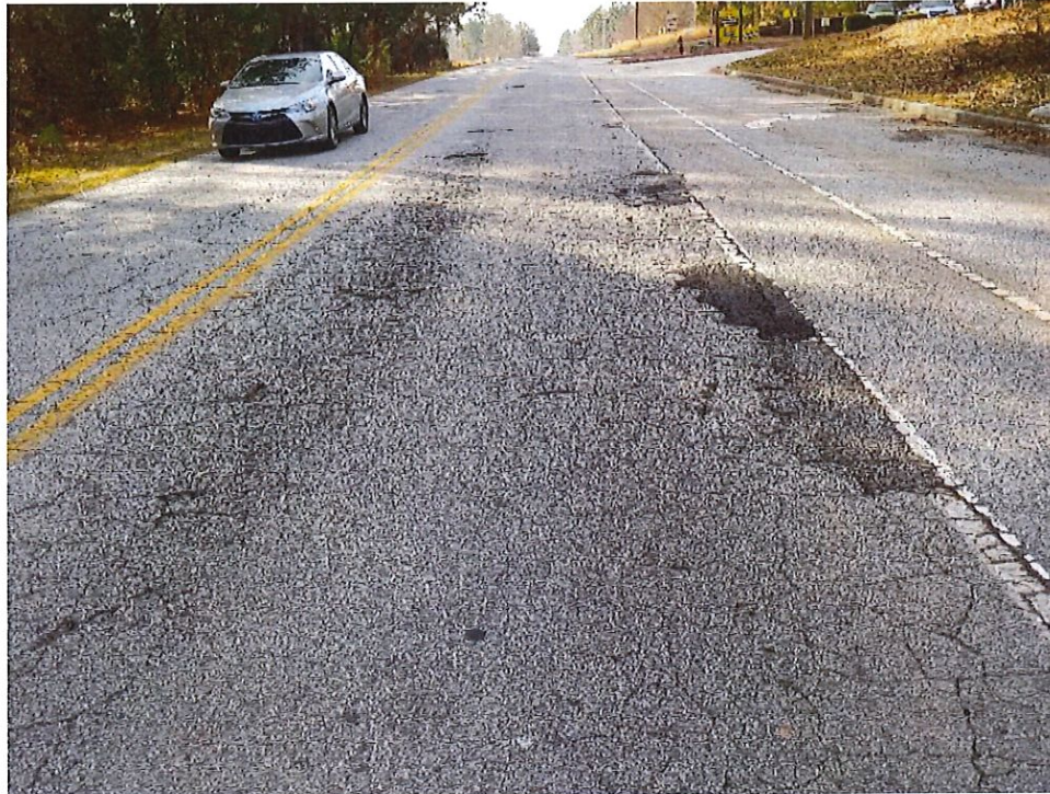
Level 4 load cracking, Southbound, Lane 1, Station 15+00±
